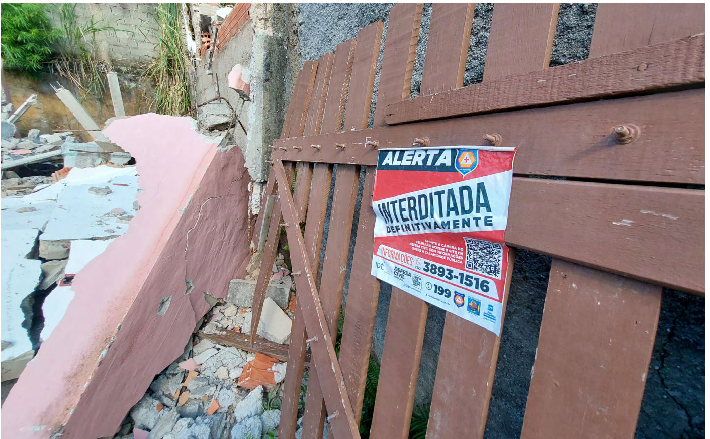
Landslide caused by the rains in Itatinga, in February 2023.
